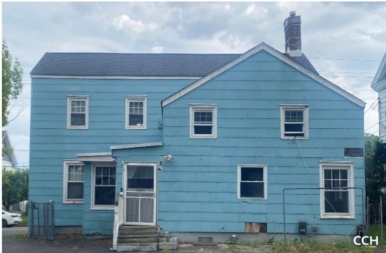
Photograph 8. Single Family House Conditions, Rear Façade.
