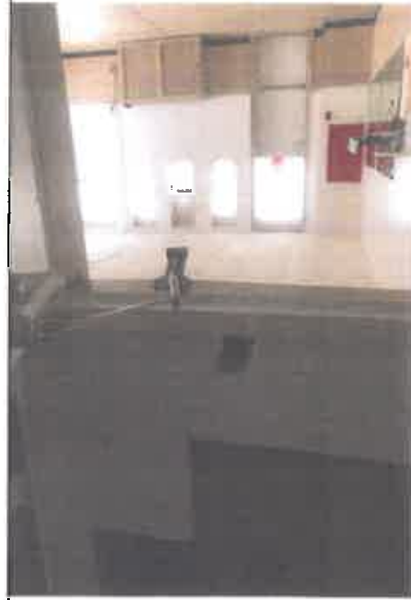
Photo 12: 2 nd Floor, Room 4
