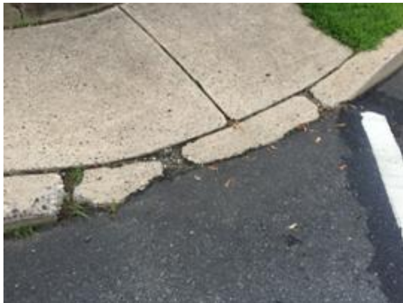
Ramp damage, SE corner
